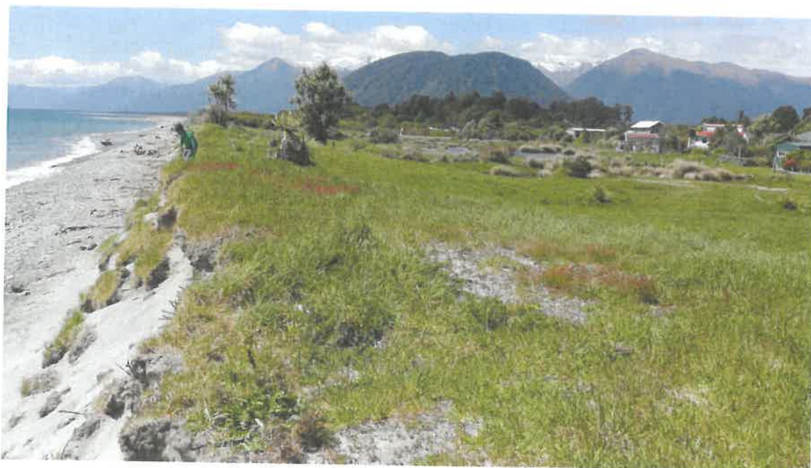
Figure 3-3: Eroding grassed-over sand-dune, Neils Beach settlement. View east towards Arawhata River mouth.
